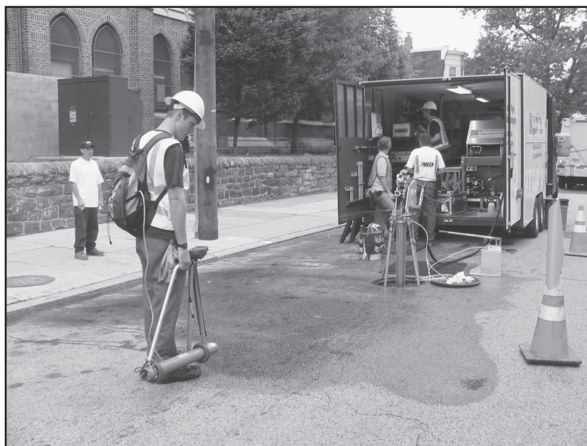
Figure 5-6 Use of inline leak detection technology in a 48-in. water main (Courtesy of Philadelphia Water Department)
