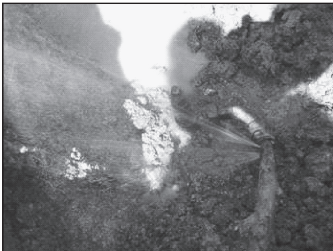
Figure 4-3 Small leak on customer service connection piping
