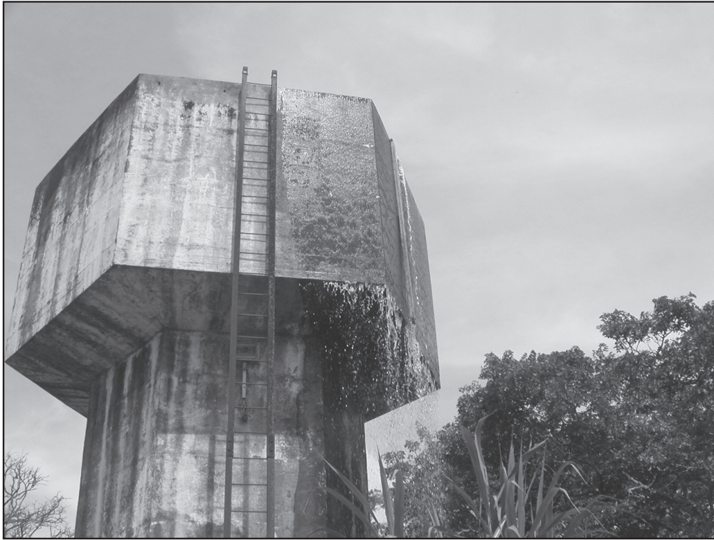
Figure 4-1 Tank overflows are a component of real losses (Courtesy of R. McKenzie, WRP Pty, Ltd.)
