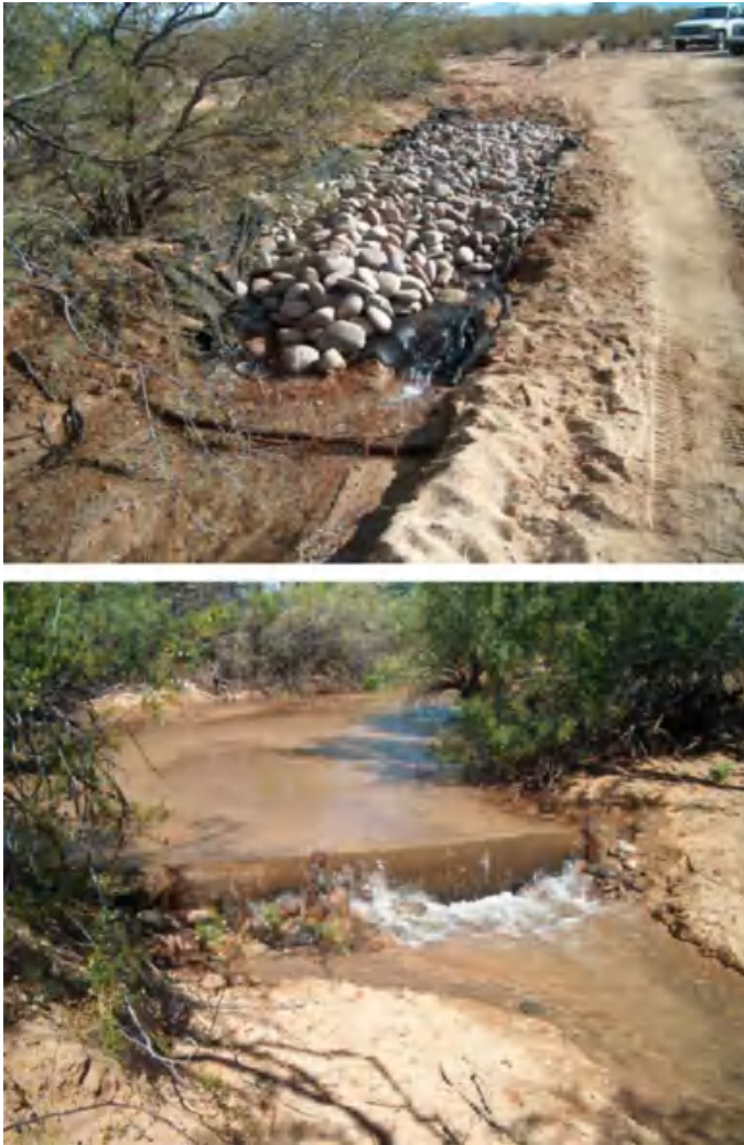
Fig. 16.2 Riprap-filled excavation discharge structure (top) and check dam (bottom) used to manage erosion during in-channel recharge, Arroyos Ground-Water Recharge Project, Pima County, Arizona ( Source USBR 2009)
