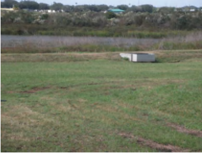
Fig. 15.4 Infiltration basin overflow outlet, Celery Fields, Sarasota County, Florida. Overflow discharges to adjoining man-made wetlands of the Celery Fields Regional Stormwater Facility
