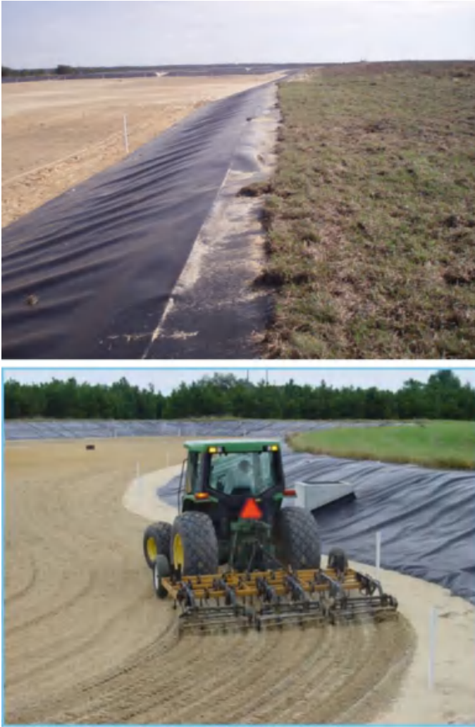
Fig. 15.9 Photographs of Water Conserv II RIBs showing HDPE geomembrane liner and maintenance (harrowing) of basins
