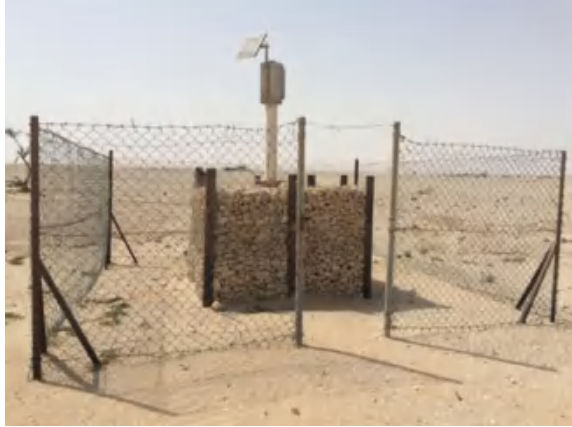
Fig. 13.7 Qatar drainage well. A perforated steel casing is surrounded at land surface by a filter consisting of gravel surrounded by a wire mesh
