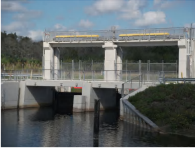
Fig. 16.4 Dam with gated spillway. South Florida Water Management District, control structure S-190, Seminole Tribe of Florida Big Cypress Reservation
