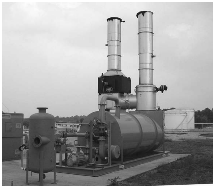
FIGURE 6-10. Large gas-fired thermal/catalytic oxidizer. (Photograph provided by Intel-lishare Environmental, Inc.)
