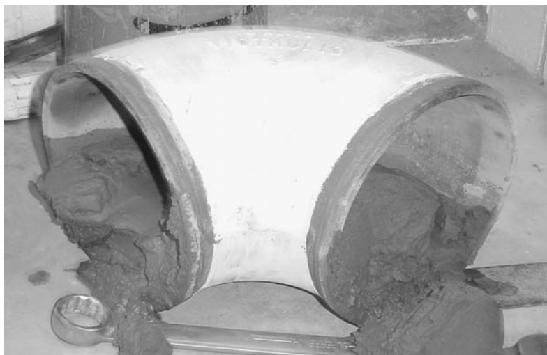
FIGURE 7-3. Silt material collected in the system piping.
