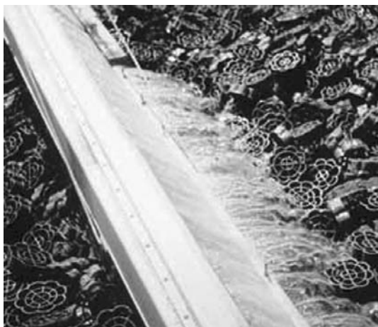
FIGURE 3-17. Photo of a rotating distributor of trickling filter with random plastic media. (Courtesy of Jaeger Environmental, www.jaegerenvironmental.com/ )
