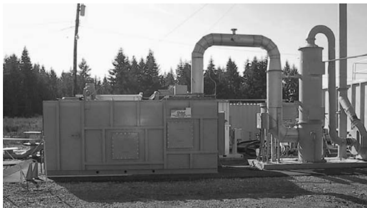
FIGURE 6-13. Catalytic oxidizer with integral scrubber. (Photograph provided by Anguil Environmental Systems, Inc.)
