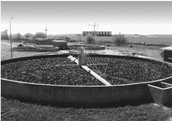
FIGURE 3-16. Photo of a trickling filter with random plastic media. (Courtesy of Jaeger Environmental, www.jaegerenvironmental.com/ )
