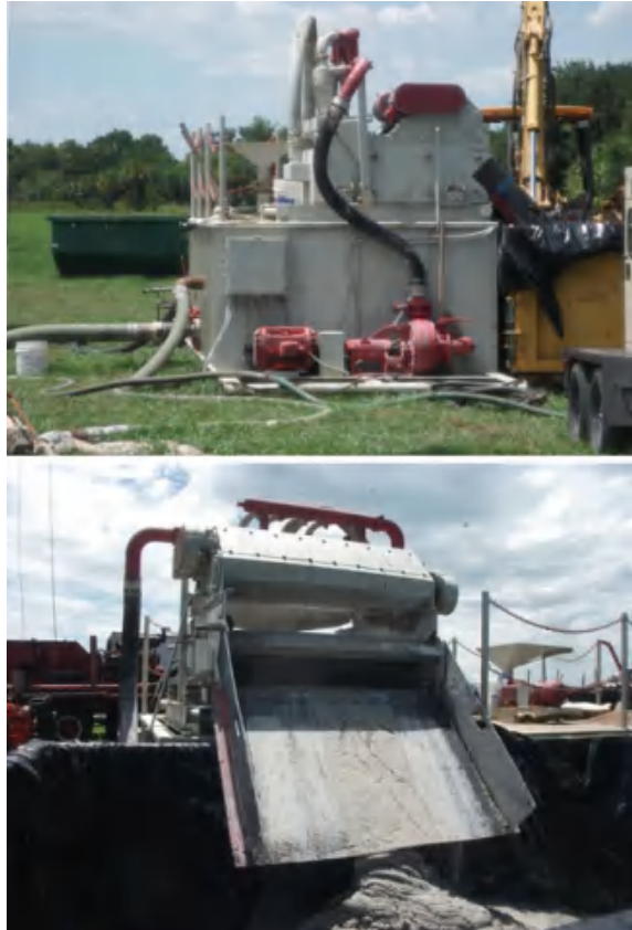
Fig. 6.6 Desanders and shale shaker used to separate cuttings from the drilling mud
