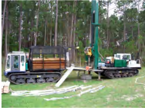
Fig. 6.9 Sonic drilling rig. Collected cores were laid out on visqueen for description and then boxed and archived
